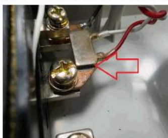
CIRCUITO DE CORRIENTE DETERIORADO (Shunt)
